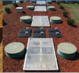
Onsite Wastewater Treatment
